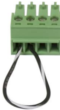
Figure 4-4: Jumper Wire Between COM Transmit and Receive Terminals
